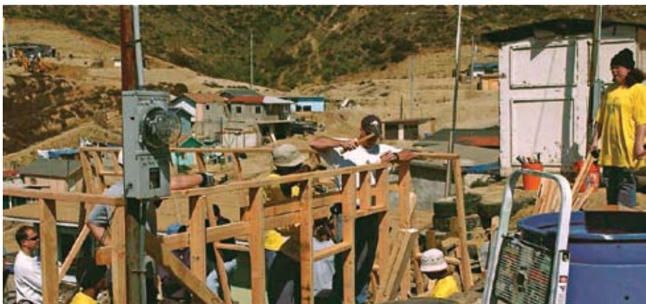
CHC staff and youth build a family a new home in Tijuana
